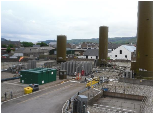
Figure 1: Campbeltown SIU, ambient vaporisers in centre
