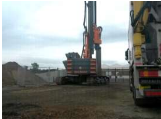
Figure 3: Bauer industrial pile driver that caused damage to main
